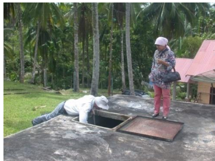
Reservoir Gasan Gadang Kap. 135 M 3
